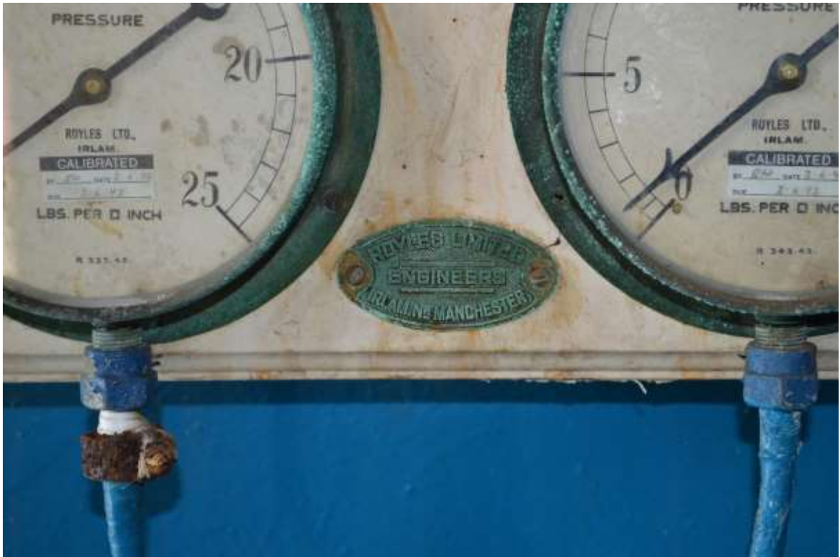
25: Royles board to cylinder outlets Nos. 1 and 2 in Northern Building, close-up.
