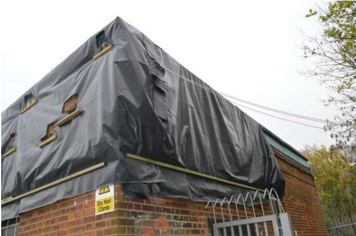
46: View of the south-western corner of the Southern Building. Note the temporary tarpaulin to the upper sections and temporary timber battens.
