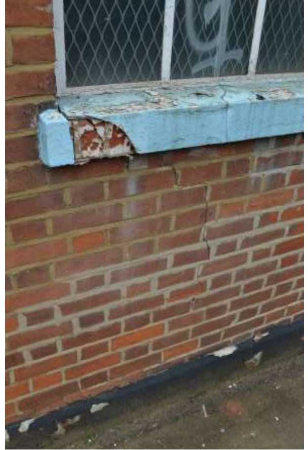
32: Lintel to most northern window on eastern elevation. Note crack to lintel and brickwork beneath.
