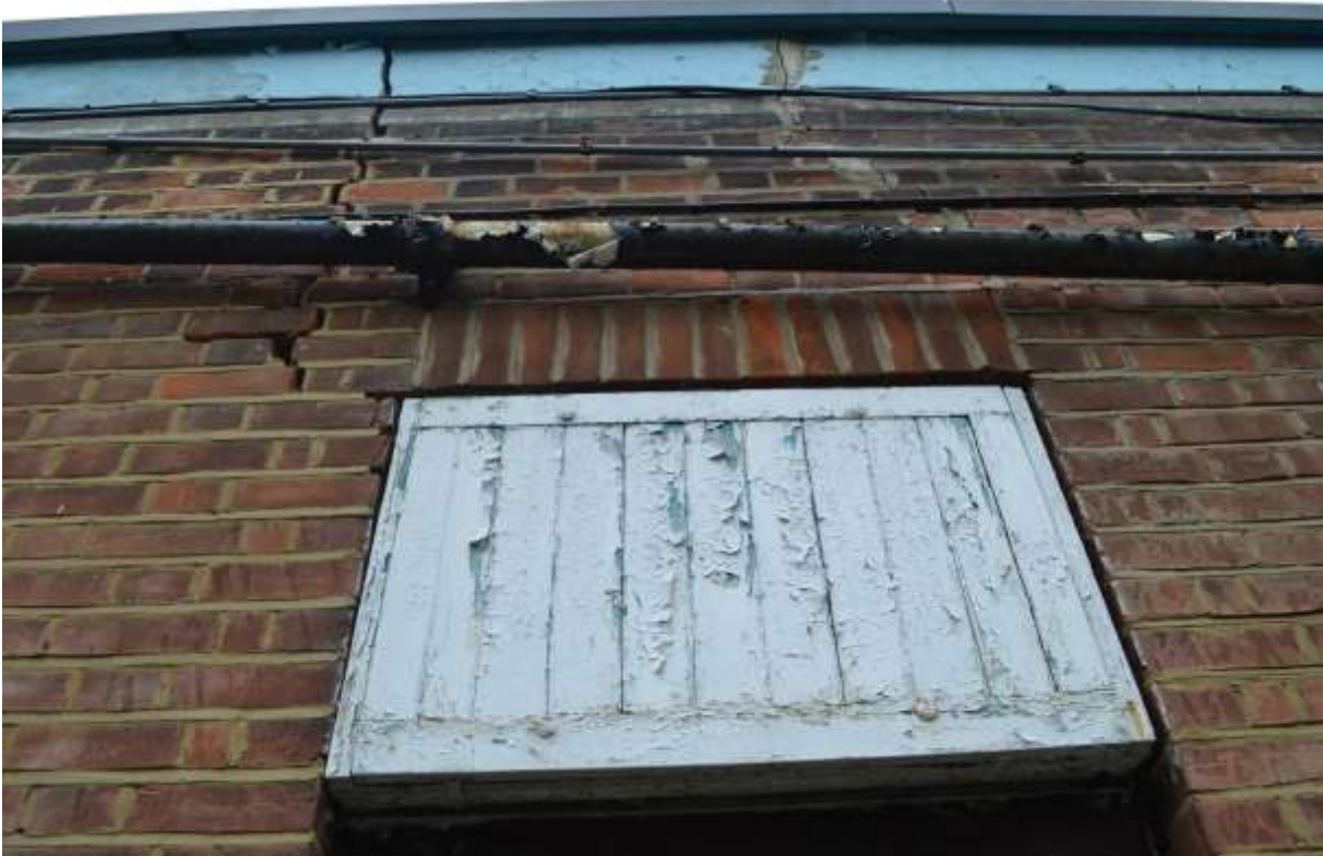
33: Upper part of central window to eastern elevation. Note the substantial crack to the upper left hand side.
