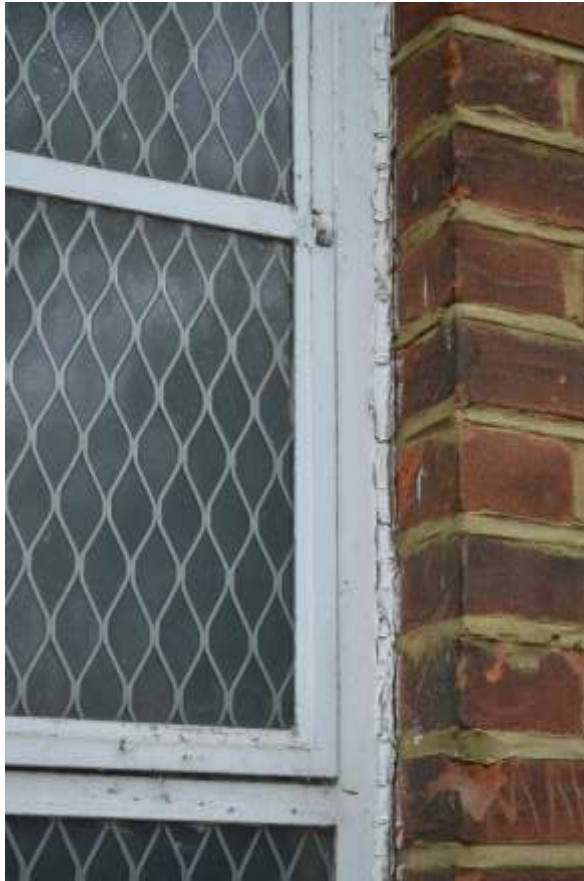
40: Close up of the central pivoting point to the steel framed window on the southern elevation.
