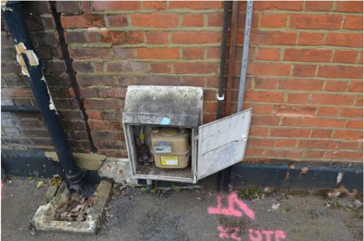
15: Gas meter on eastern elevation towards southern end.
