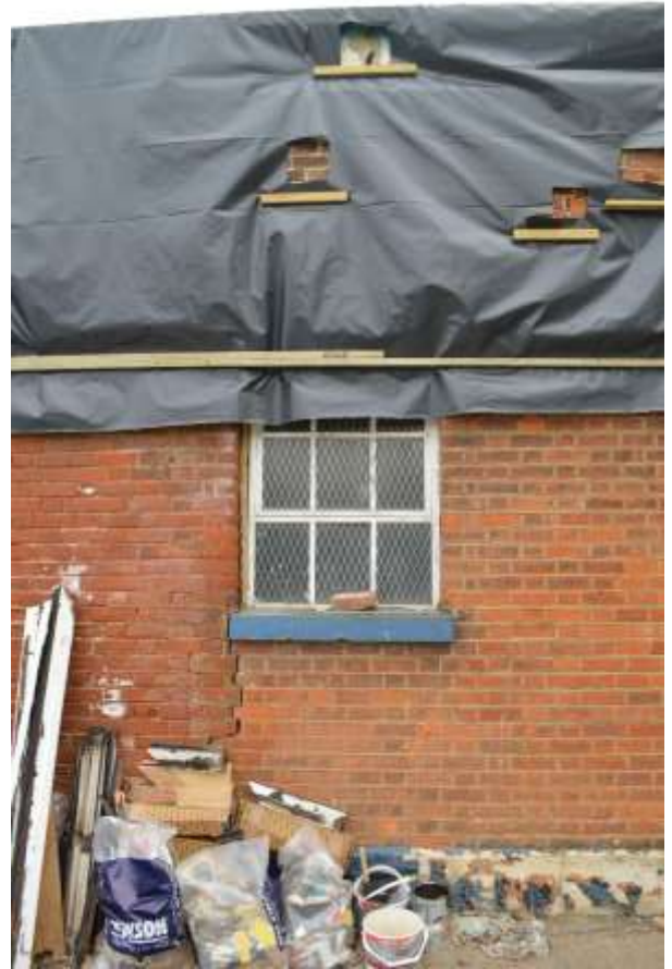
48: Note the numerous large structural cracks that have been left uncovered so that they can be monitored. Note the significant crack to the lower left side of the window cill.
