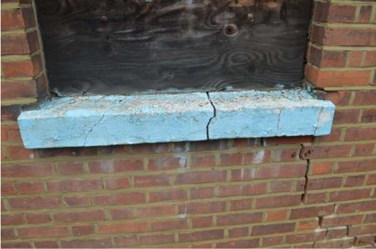
34: Lower part of central window to eastern elevation. Note the substantial crack to the lower right hand side.
