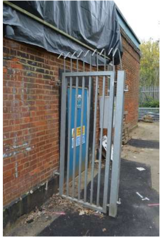
43: Modern security gate affixed to the southern elevation.
