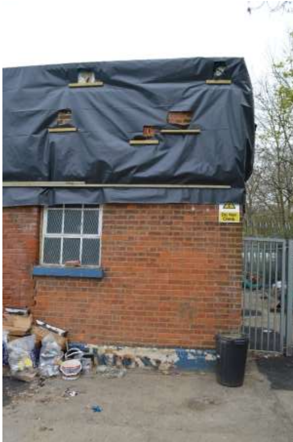
47: Southern end of the western elevation. Note the tarpaulin to the upper sections and the temporary timber batten.
