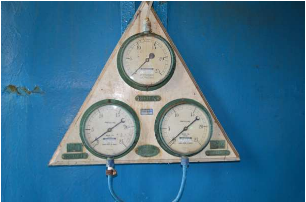
24: Royles valve board to Cylinder Outlets Nos. 1 and 2.
