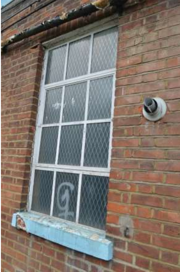
31: Most northern window on eastern elevation. Note modern flue to the right hand side.
