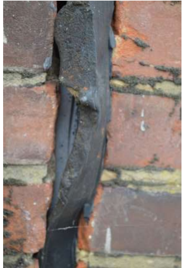
18: Infill material between Northern and Southern Buildings. Note polystyrene behind and also brickwork between the two buildings not bonded in.
