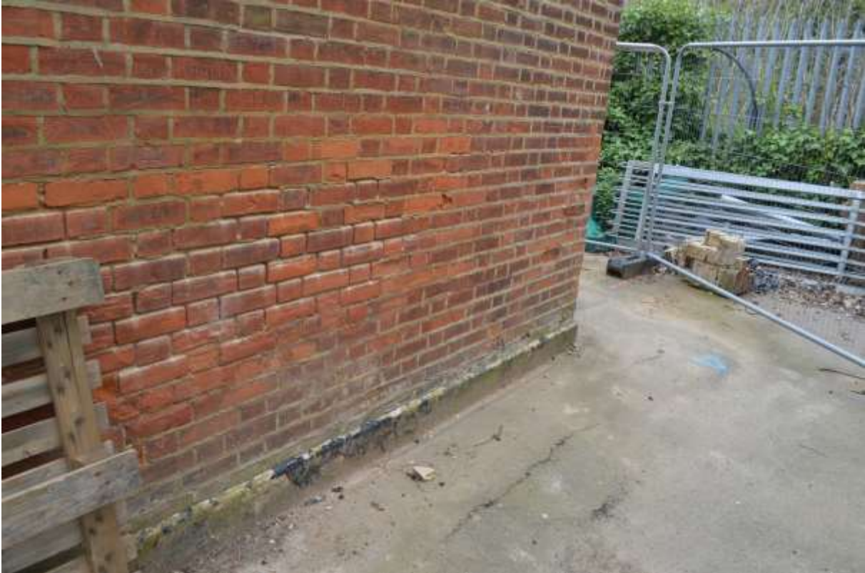
44: Pointing degradation on part of the southern elevation and brickwork spalling.
