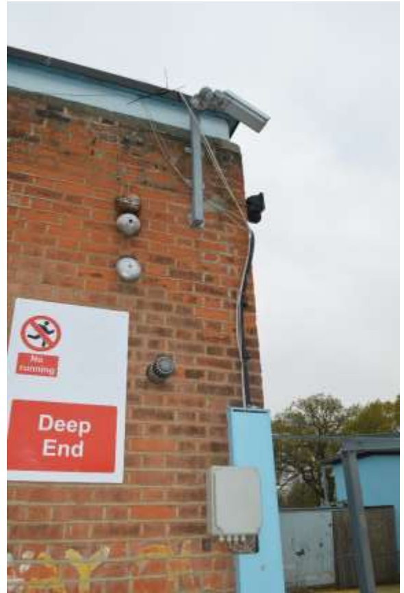
10: Security camera and conduits to north-western corner of Northern Building.
