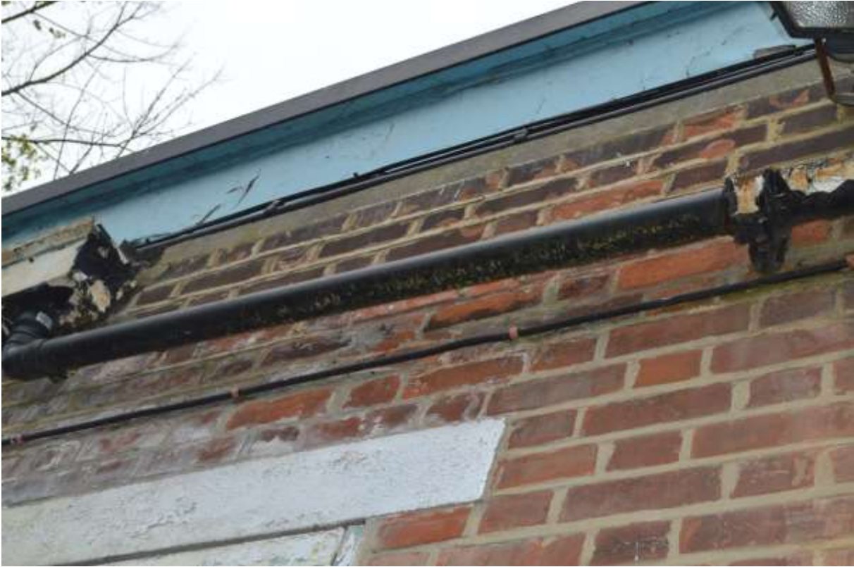
36: First section of downpipe is low grade uPVC, at southern end of the eastern elevation.
