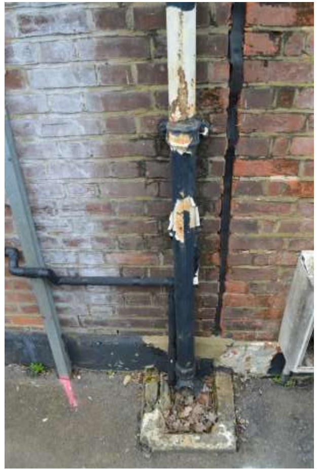
29: Cast iron hopper and downpipes at the northern extreme of the eastern elevation, lower section.
