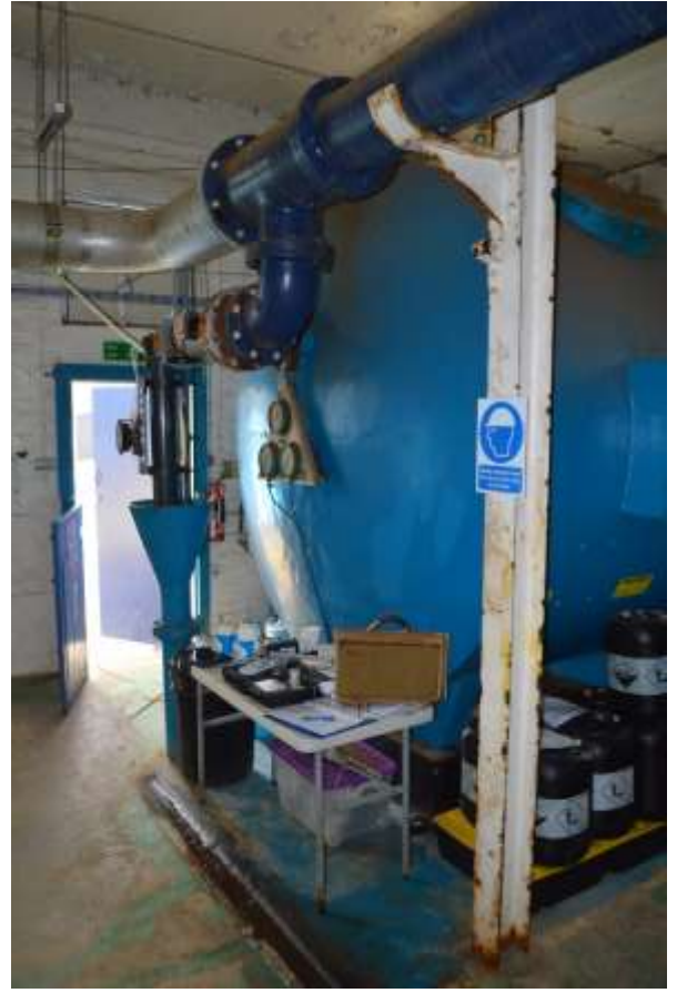
23: Royles cylinder No. 1 close to front entrance door.
