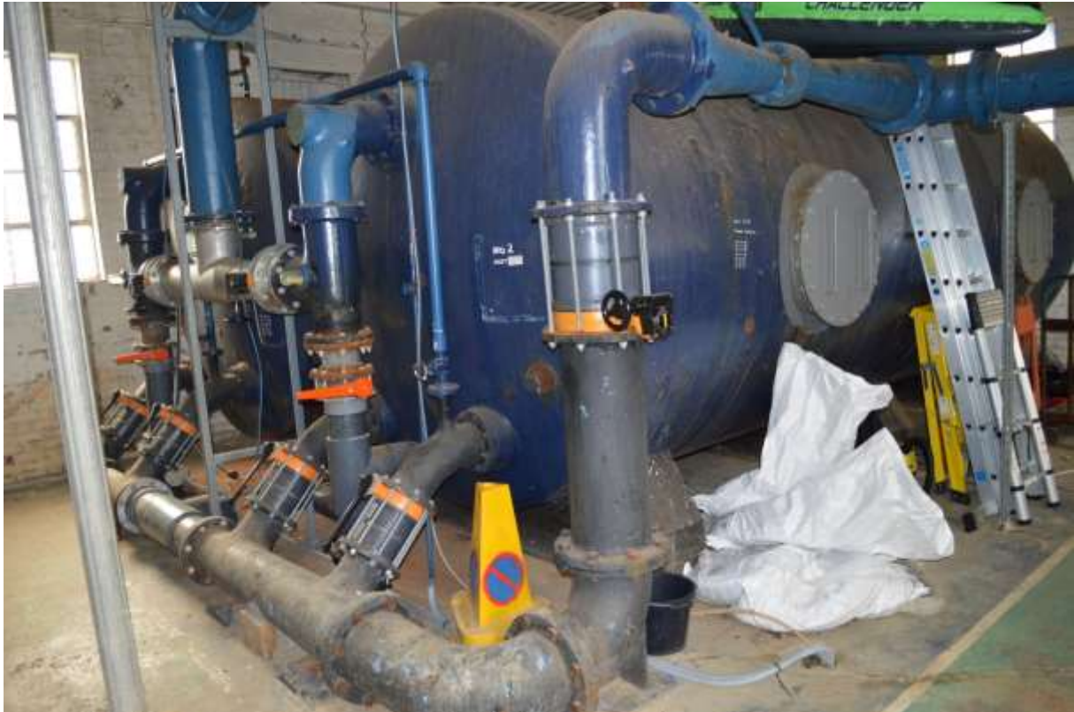
56: Showing Cylinder outlets 1 and 2 in the Southern Building and a plethora of historic pipework.
