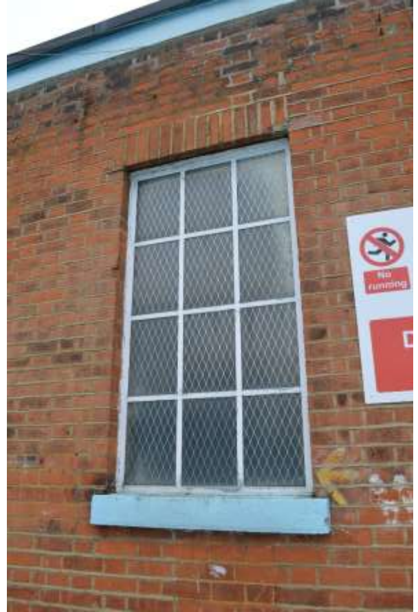
8: Western later window to front elevation. Note no steel loops to glazing bars.
