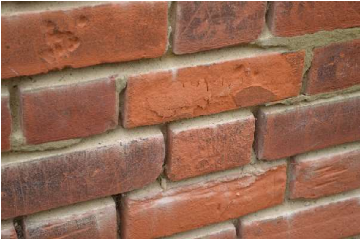
45: Pointing degradation on part of the southern elevation and brickwork spalling.
