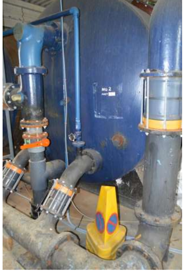
58: Close-up photograph of Cylinder outlet No. 2.
