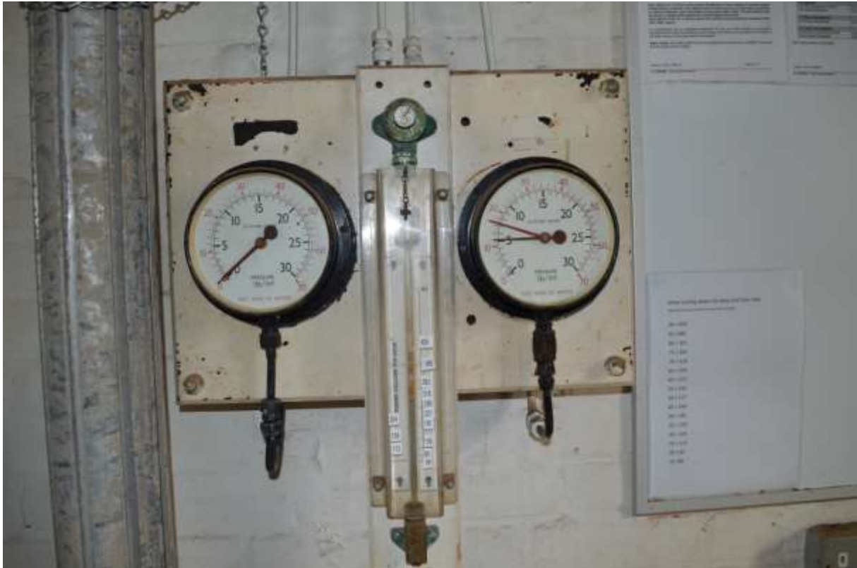
61: Valve board for Cylinders Nos. 1 and 2 on the party wall between the Northern and Southern Buildings. Historic and likely original to the construction of the Southern Building.
