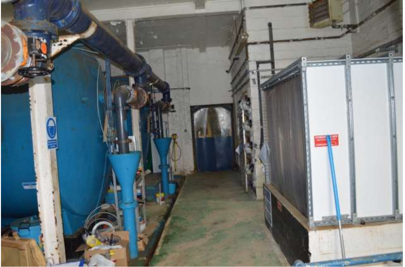
26: View looking south through the Northern Building towards the dividing door between the Northern and Southern Buildings.
