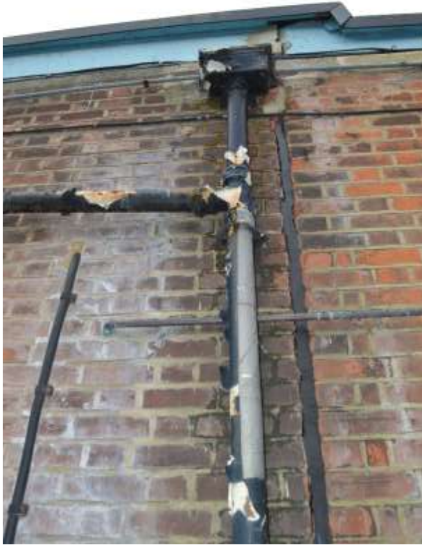
28: Cast iron hopper and downpipes at the northern extreme of the eastern elevation, upper section.
