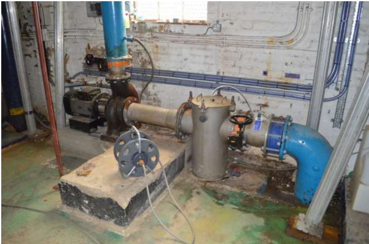
62: Historic pipework, valves and plant in the north-western corner. Also modern plant to the left hand side.
