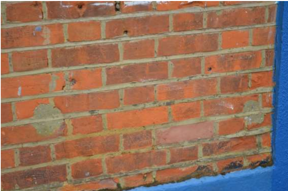
4: Section of poor quality pointing to the left hand side of the main entrance, above plinth render. Also showing mortar repair to one brick.
