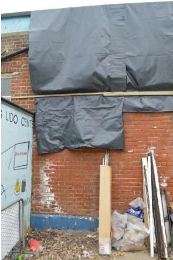
51: Middle section of the western elevation between the two windows. Hoarding to the left hand side.
