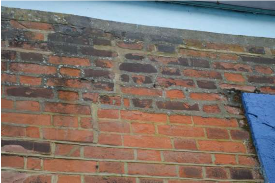
3: Section of poor quality pointing to the left hand side of the main entrance, above door architrave.
