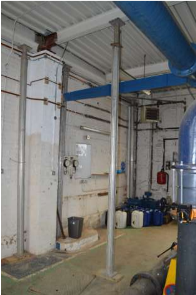
53: View of the north-eastern corner of the Southern Building. Note the Acrow props supporting the roof and the I-beams.
